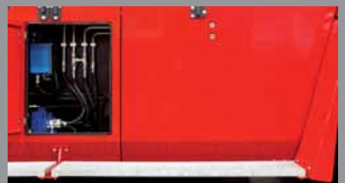
Pressurized Hydraulic Oil tank
