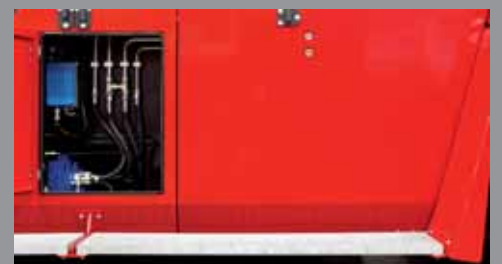
Pressurized Hydraulic Oil tank
